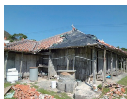
(c) Partially Damages
