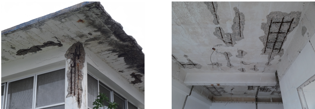
FIGURE 13. Concrete deterioration due to salt content
