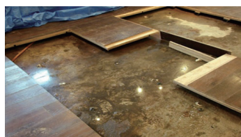
(e) Inundation under the floor level
